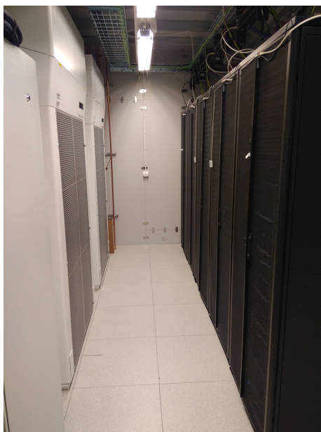
Figure 3: Photo of the space that lies between the CRACs and the servers for the system that we used in our experiments.
